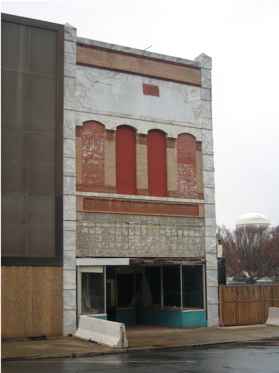
Figure 5. General condition of many of the downtown buildings.
